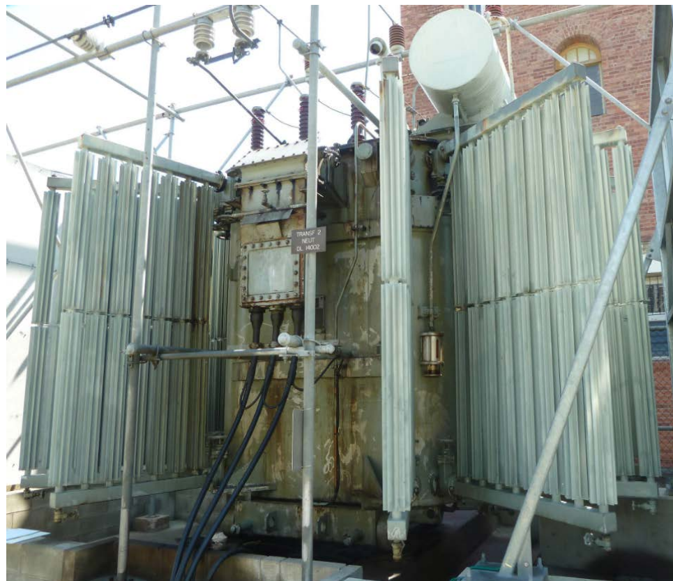
Figure 8: 5MVA 33/5.5kV Transformer TR2
