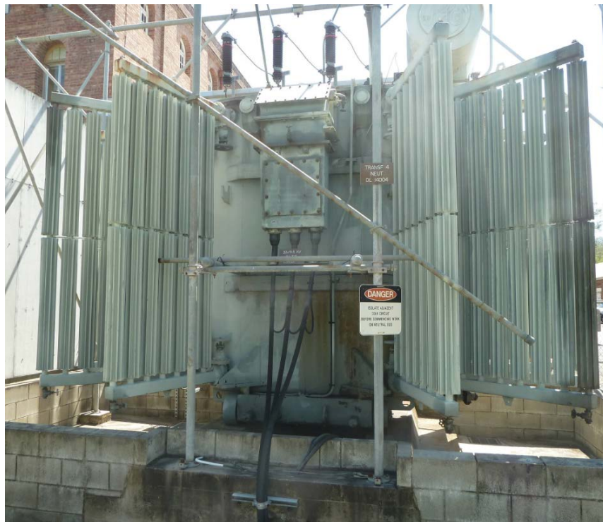
Figure 10: 5MVA 33/5.5kV Transformer TR4
