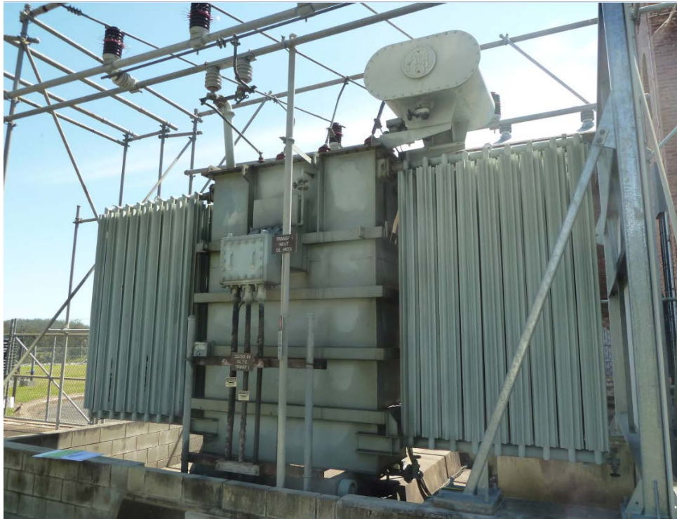
Figure 7: 5MVA 33/5.5kV Transformer TR1
