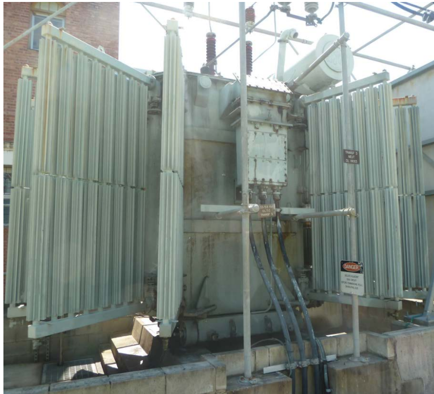
Figure 9: 5MVA 33/5.5kV Transformer TR3
