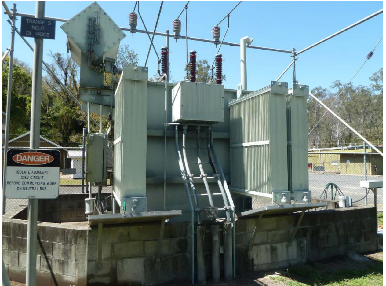
Figure 11: 5MVA 33/5.5kV Transformer TR5
